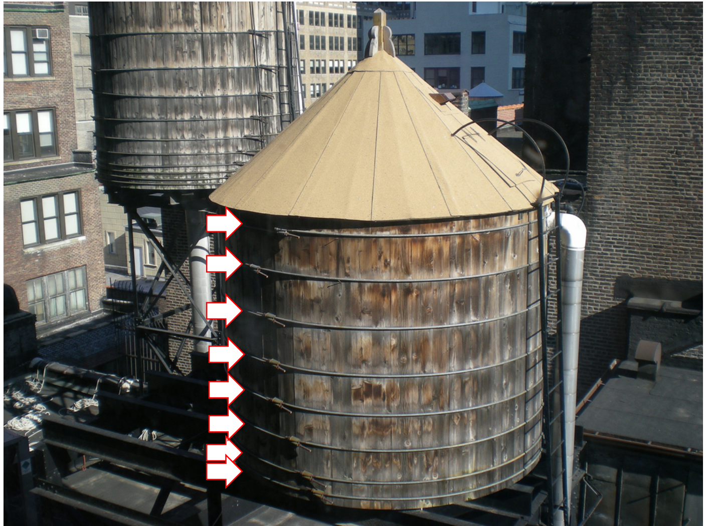
Domestic water storage tanks in New York City
